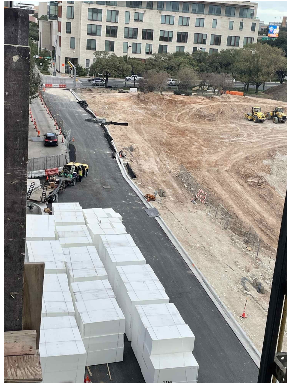
View facing North towards Dell Medical School of new Red River Street
